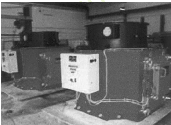
Fig. 13.1 Double chamber incinerator (Capacity: 2 × 800 kg/day)
